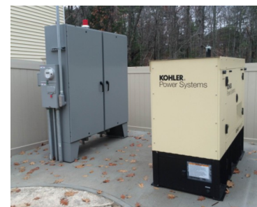
The new and improved Powder Mill pumping station. New pumps, controls and a backup generator were installed as part of the upgrade.
