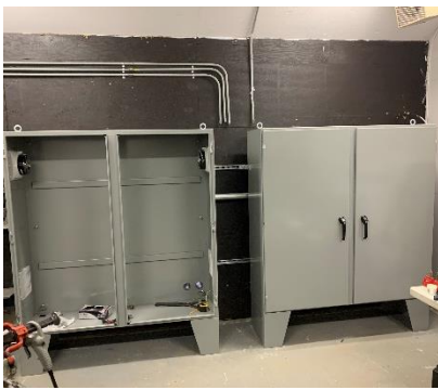
Riverlocks 1 Control Panel Upgrade
