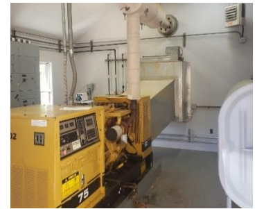
Lakebrook pump station
